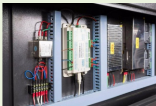
Perfectly Tidy Power Supply System
